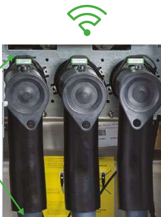
TH110 sensors mounted on cable connections
