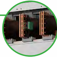
Main Busbar joint
